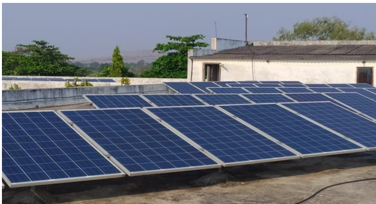
SOLAR Grid connected solar plant (15.3KWh)
