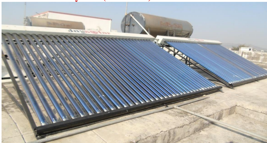
Solar Water Heater System (2000 LPD)
