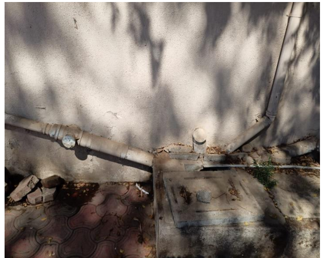
Sewer for wastewater from toilet at Main building
