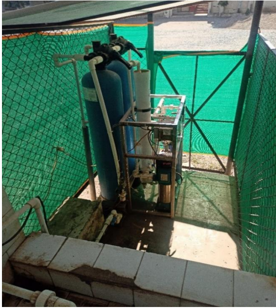
3. Water Purifier System in College campus
