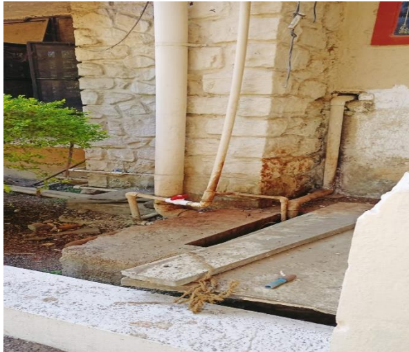
Drainage system of Chemistry department
