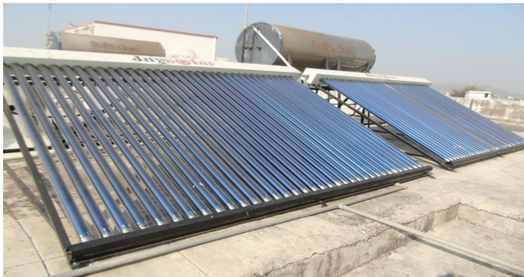
Solar Water Heater System (2000 LPD)
