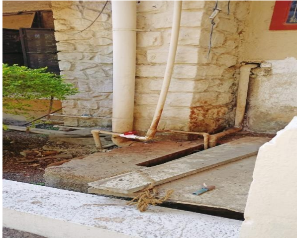
Drainage system of Chemistry department
