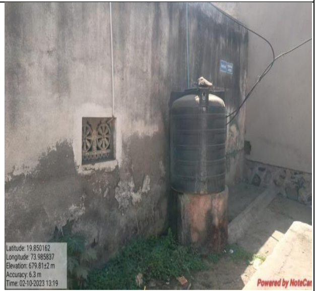
Storage Tank Near Canteen
