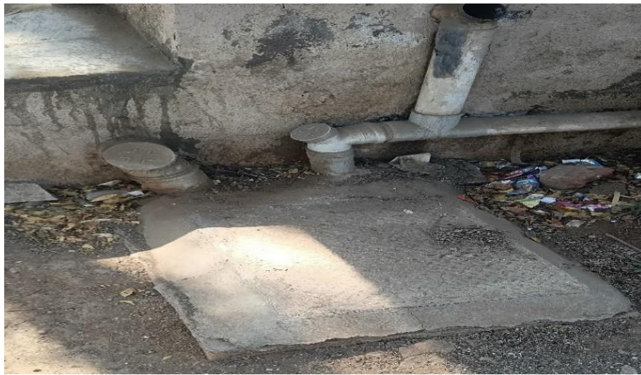
Septic tank near toilet of main building
