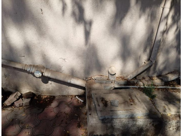
Sewer for wastewater from toilet at Main Building
