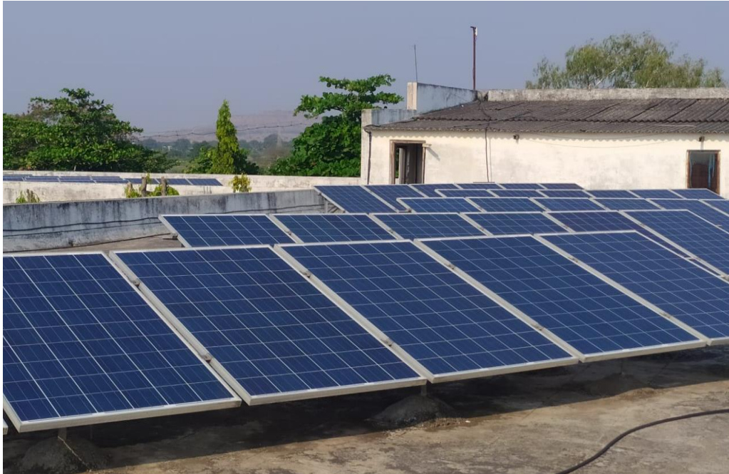
SOLAR Grid Connected to Solar Plant (15.3 kWh)
