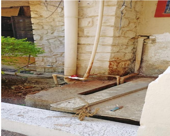
Drainage system of Chemistry department
