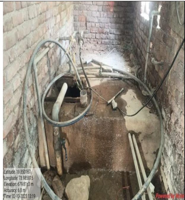
Water Storage Tank
