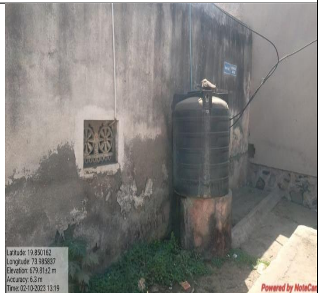
Storage Tank Near Canteen
