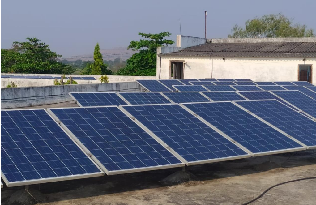
SOLAR Grid Connected to Solar Plant (15.3 kWh)
