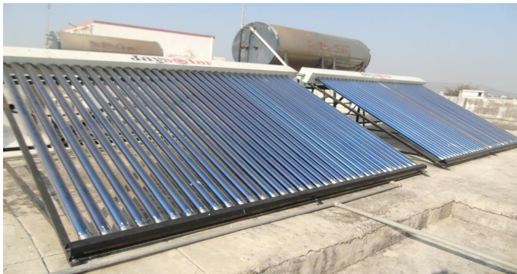
Solar Water Heater System (2000 LPD)
